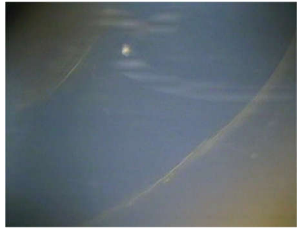
Pipe Implosion Identified
