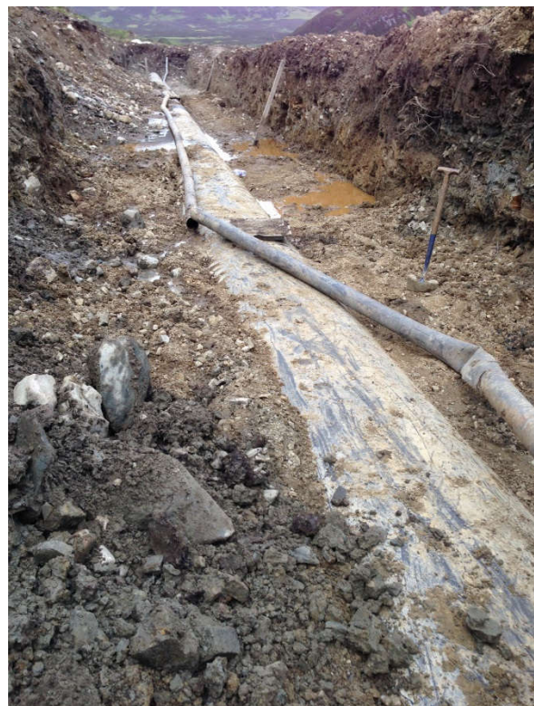
Exposed Imploded Pipeline
