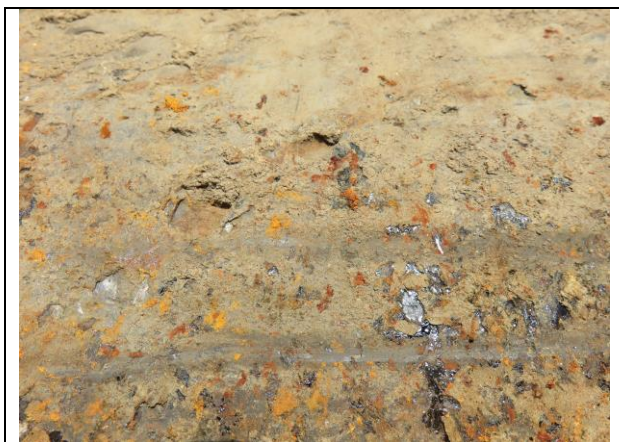
Pipe wall image pitting
