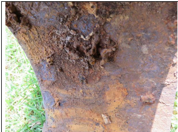
Pipe wall image tuberculation identified
