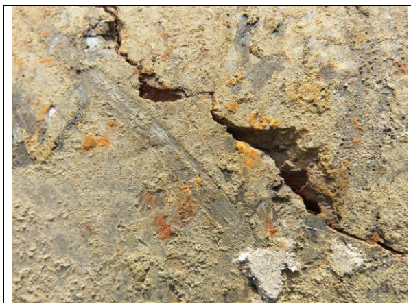
Pipe wall image fracture
