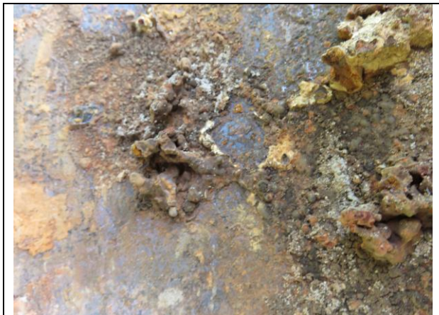
Pipe wall image tuberculation identified
