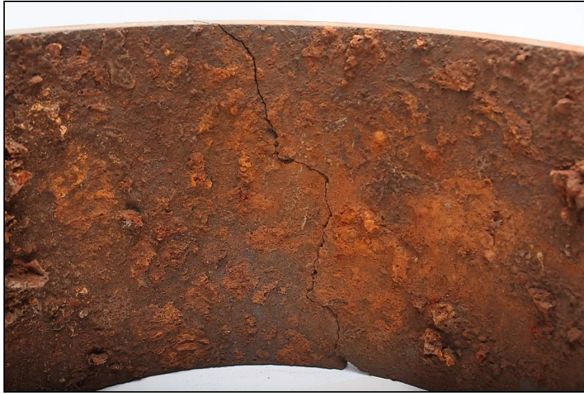
Figure 2: The main crack through the section of pipe provided.
