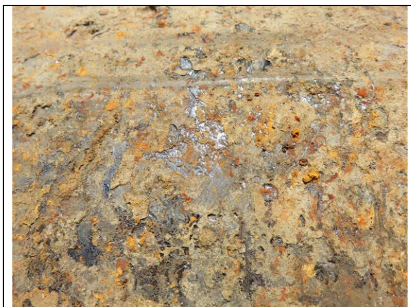
Pipe wall image
