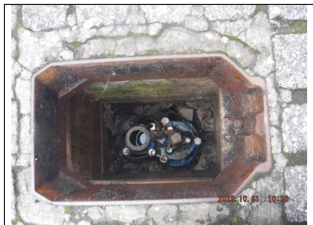
Camera insertion point hydrant
