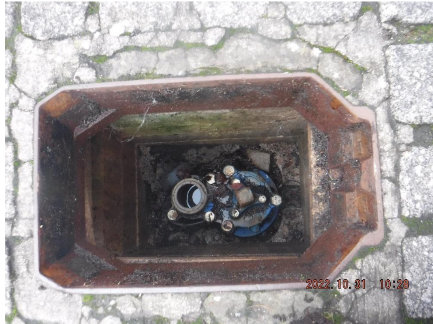
Image of hydrant bowl condition
