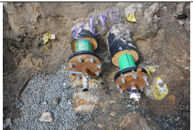
Pipepod insertion point:
