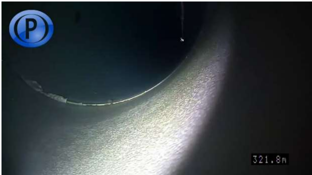
Debris on joint image
