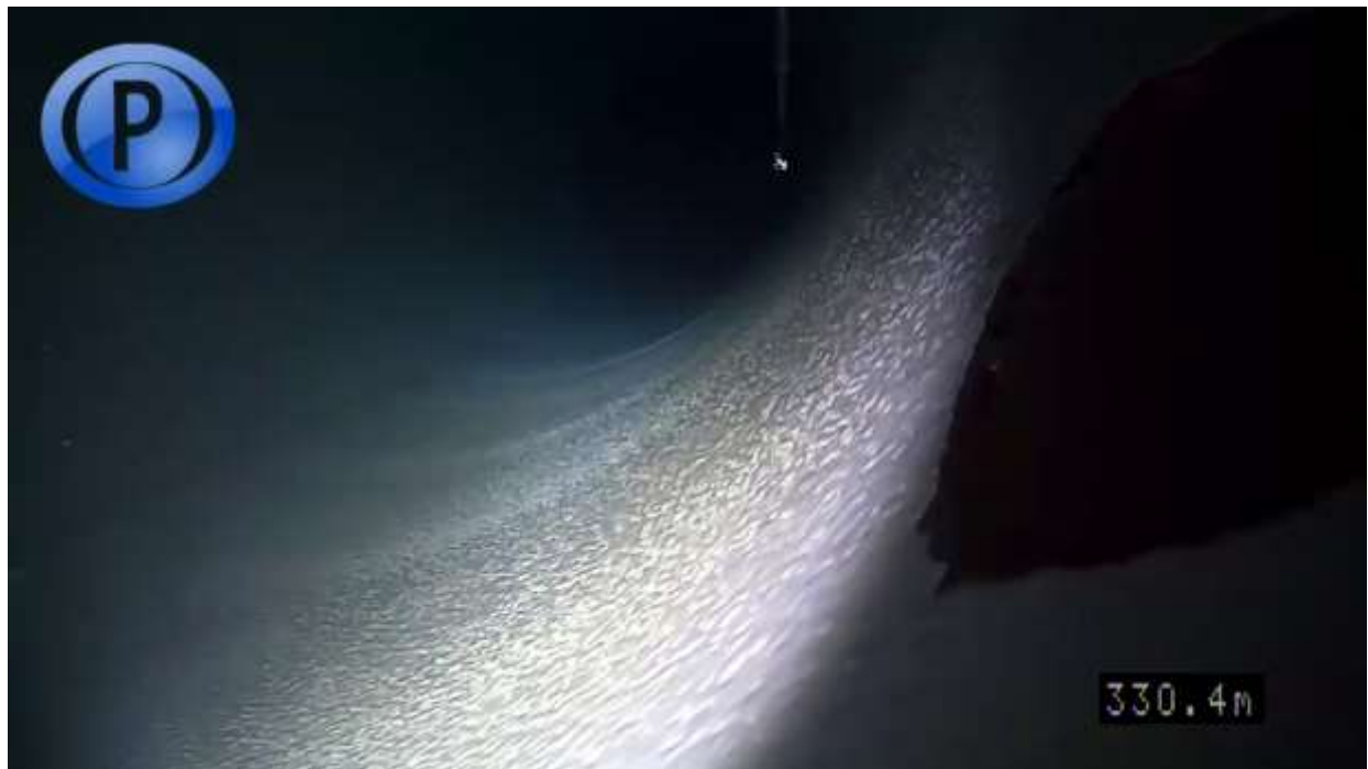
Possible failure of cement lining
