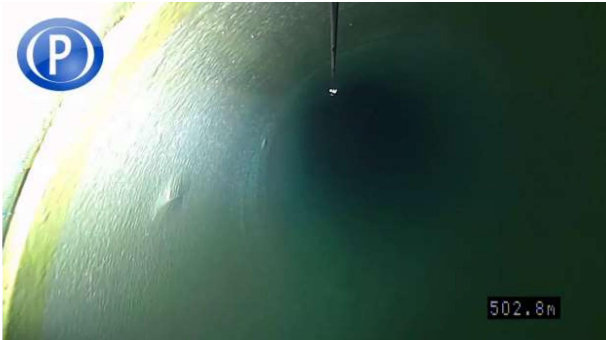
Main image with blistering of lining identified
