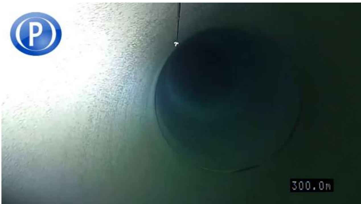
Joint image possible gasket and wide joint (this point recorded an acoustic POI)
