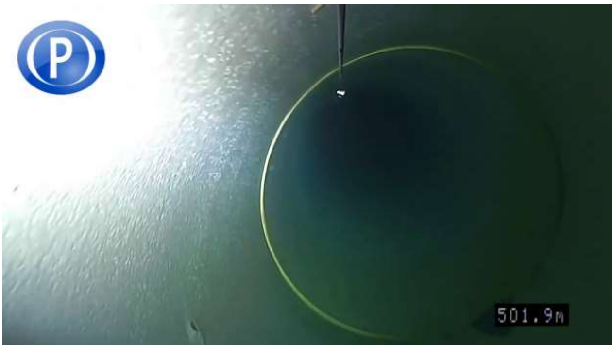
Joint image with failure of lining identified
