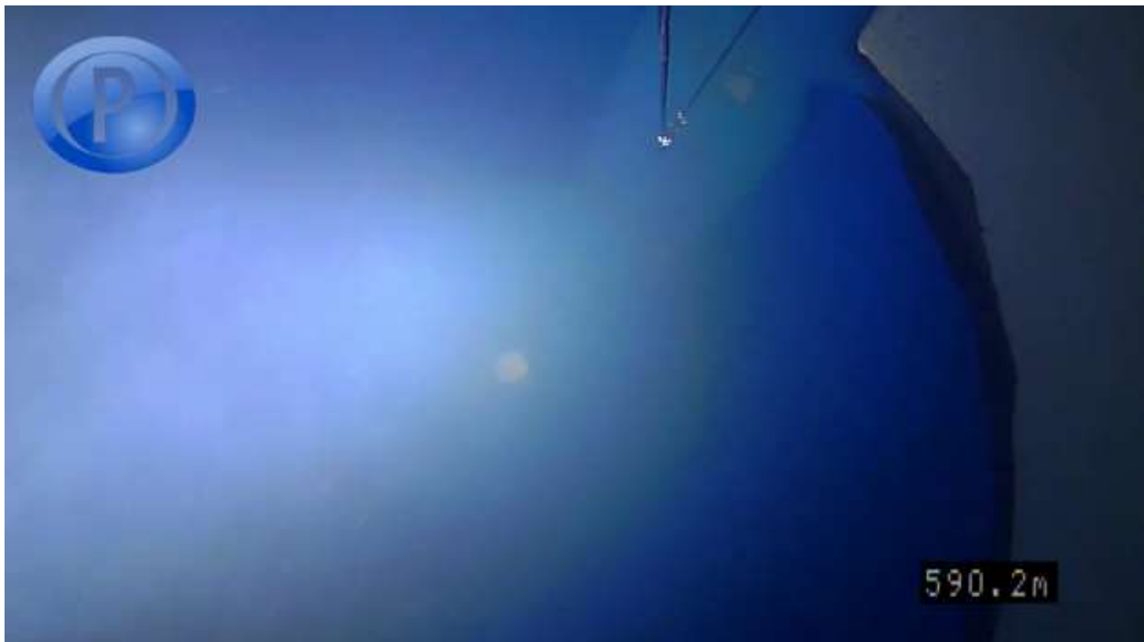
Wide joint at exit point identified
