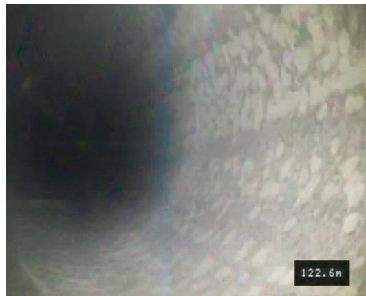
Pitting of cement lining identified
