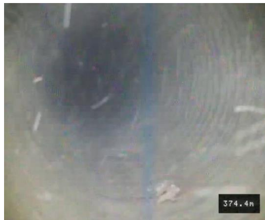
Debris in pipe identified
