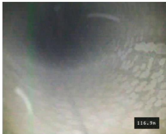
Pitting of cement lining identified
