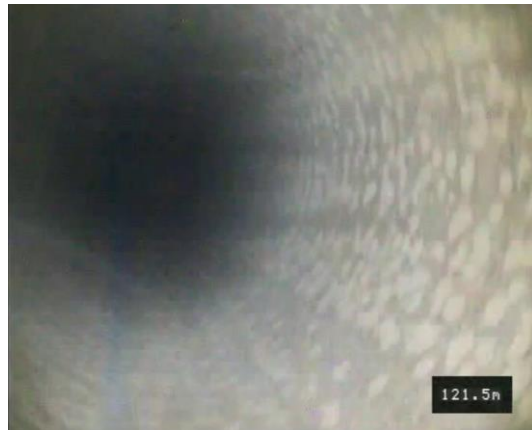
Pitting of cement lining identified
